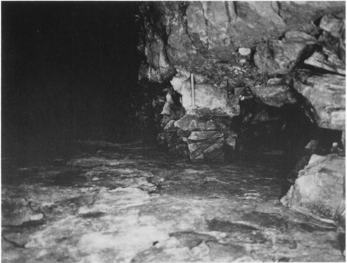
Plate 1a: Crawstone Ironstone mine in Ironbridge, abandoned in the early 19th century. Longwall workings (left) have been packed with sandstone to prevent collapse because of the adjacent roadway (right). The latter is 1.7 m high and has been sunk lower than the ironstone level to provide headroom. The low passage through the sandstone packing (left) leads to the advancing working face. (Photo: British Geological Survey).
